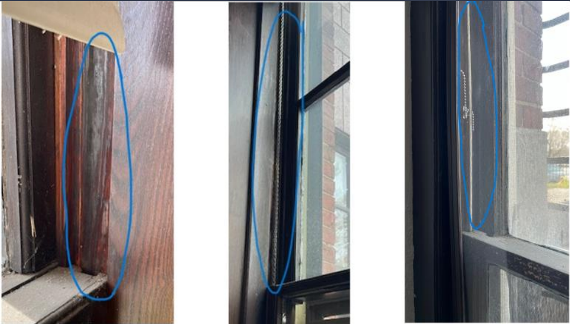
Three different window sashes in the building, ancient and inefficient
