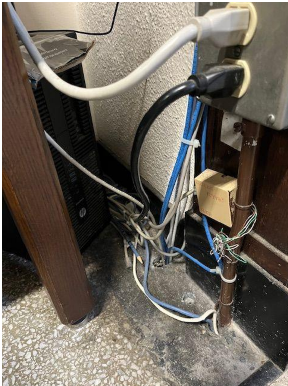
One example of the cabling situation throughout the library
