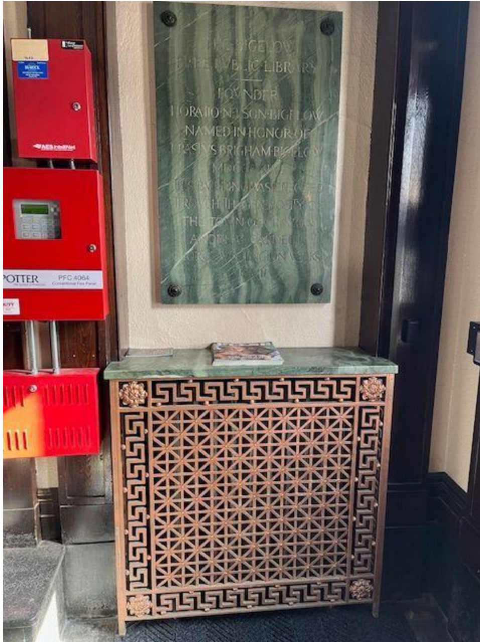
Dedicate marble and radiator cover in the front entryway with fire alarm system
